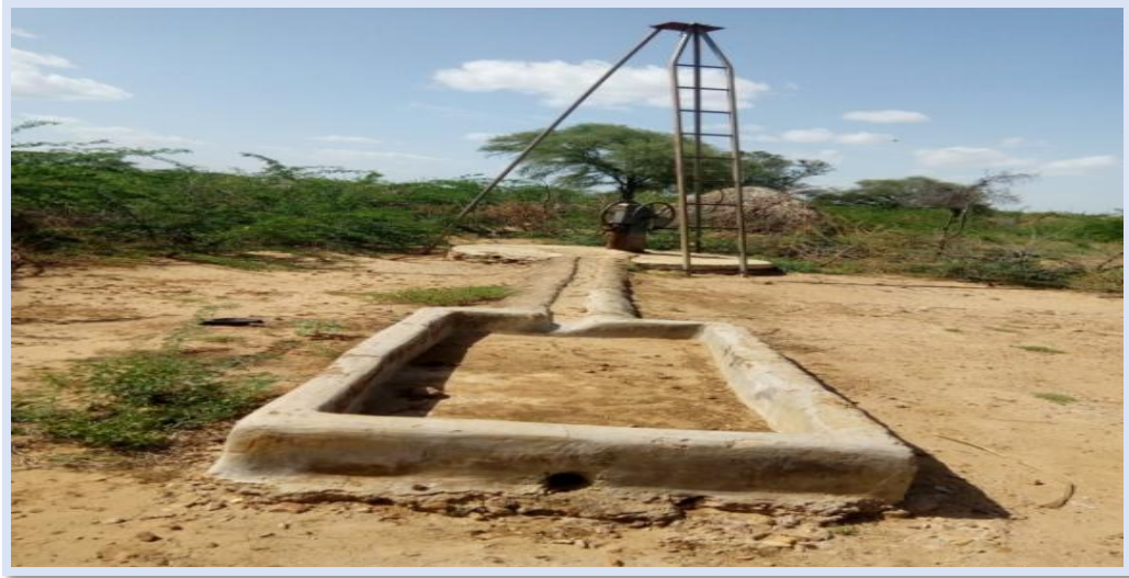
Nanam centre water supply Construction of 2 Water Tanks, 2 water kiosks and Piping GPS: (E) 465905 (N) 673270
