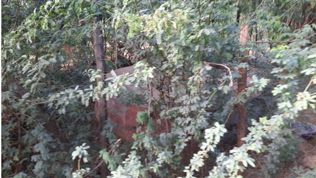
One of the four targeted boreholes in Lokariwon construction of overhead tanks connected to 4 boreholes GPS: (E) 465487 (N)649660
